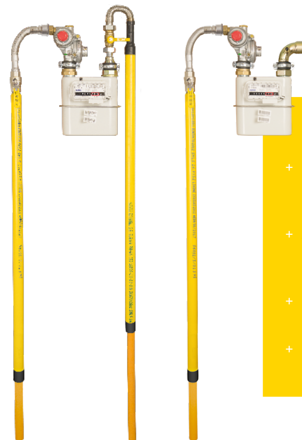
OUTLET PIPE GOING TO THE GROUND
